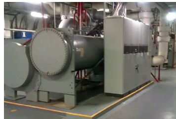
Centrifugal chiller in situ in plant room at Citi's headquarters.
