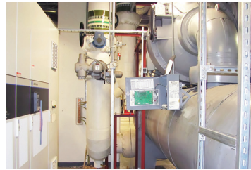
The VSD installation was delivered in sections then re-assembled in the plant room.
