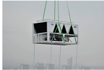
AquaSnap chiller suspended above the London skyline.
